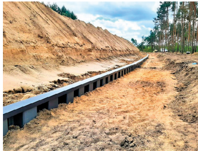
Fig. 6. Vertical waterproof barrier with PVC sheet piles installed in subsoil along waterside toe of the levee (photo Pietrucha company).
