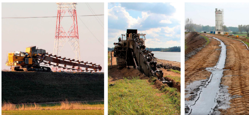
Fig. 8. Continuous Deep Soil Mixing (CDSM) method (A) Trencher on the levee, (B) Trencher during cut-off wall construction, (C) Constructed cut-off wall with CDSM method ( www.dabi.com.pl ).
