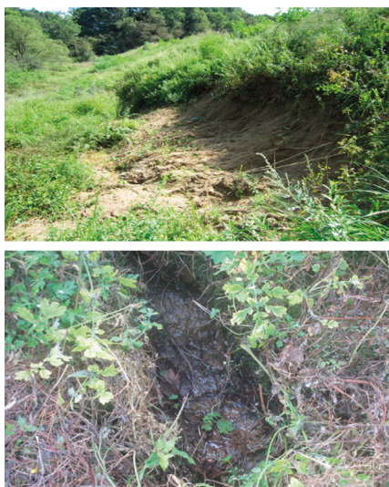
Fig. 1. Failure examples of small agriculture reservoirs and dams: (upper) slope sliding failure; (down) water leakage through down slope.
