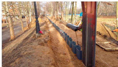
Fig. 7. Vertical waterproof barrier with PVC sheet piles installed from the crest of the levee using reusable steel cover (photo Pietrucha company).
