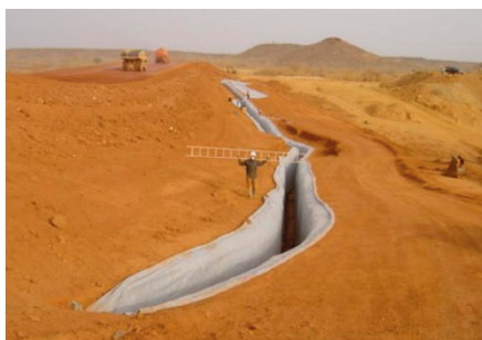
Fig. 5. Construction of a drainage ditch in the landside toe of the levee [photo Olivier Artière; CFBR 2021].
