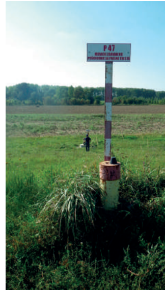
Fig. 8. Observation well with installed datalogger
