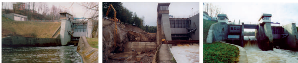
Fig. 10. WS Skalka – before and during the construction of a new spillway [photo by Vlk]
