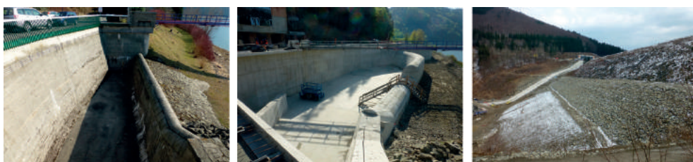
Fig. 13. WS Šance – from left: original and new safety spillway, agitating bench [photo by Kantor]
