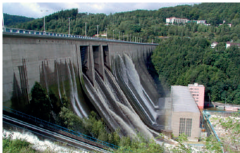
Fig. 1. WS Orlik – water discharges through ventilation openings on the air face during the flood in August 2002; the interior of the dam and the power plant were flooded [photo by D. Richtr]
