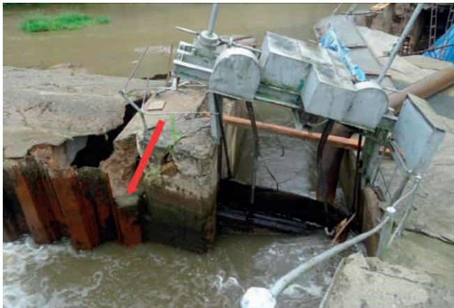
Fig. 6. The detailed view at the collapsed right sluice pier with sunk sheet pile
