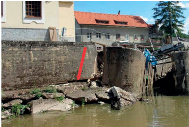
Fig. 9. Cracked toe of the right bank wall (upstream view)
