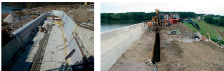
Fig. 12. WS Těrlicko – reconstruction of the safety spillway and fallout, increase of dam crest by reinforced concrete breakwater and interconnection of dam seal [photo by Rainer]
