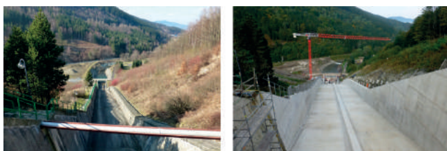
Fig. 14. WS Šance – original and new chute from safety spillway [photo by Kantor]
