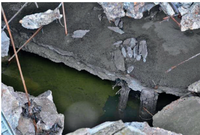
Fig. 10. Piles supporting the undermined foundation slab of the HPP inlet
