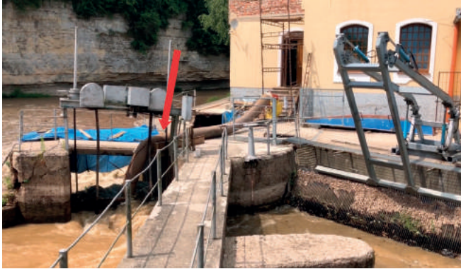
Fig. 5. The downstream view at the sluice, the arrow indicates subsidence of the backfill and platform behind the right sluice pier
